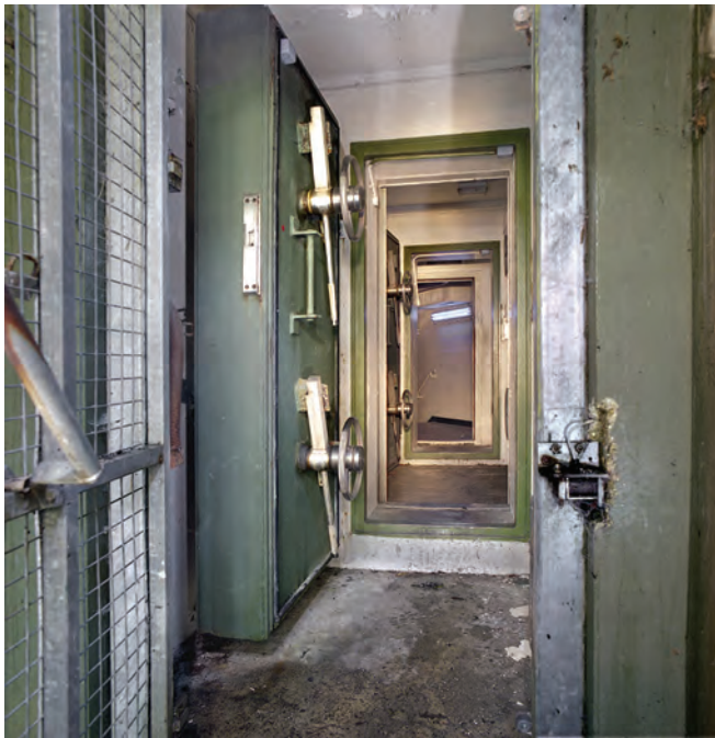
The massive blast doors in the 'clean' entrance to the bunker. Photo Nick Catford
